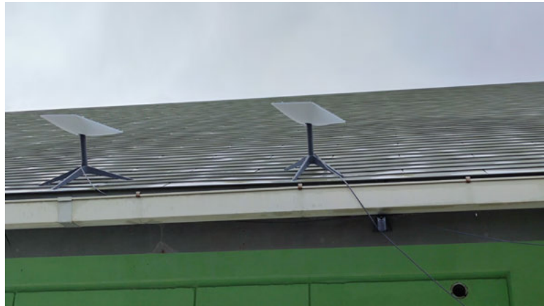
Starlink antennas on the roof of the Parliament of Kiribati. © IPU/CIP
