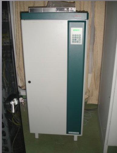
CENTRAL 40 KVA UPS
