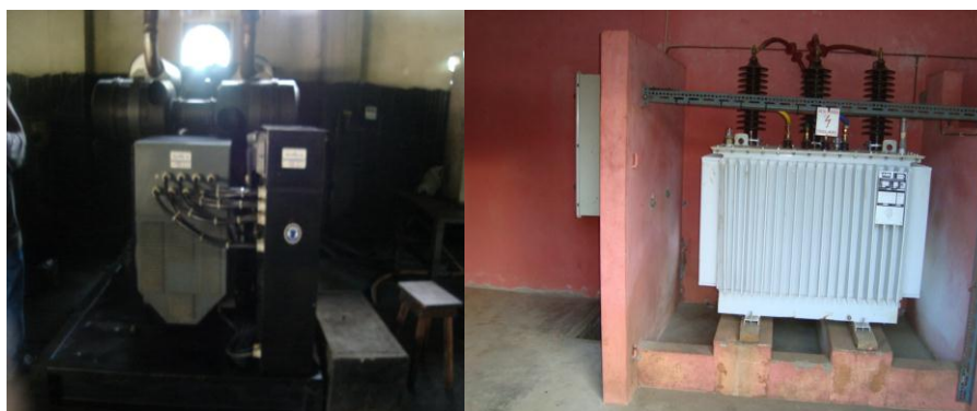
(Genset and Transformer in Inhambane Mozambique)
